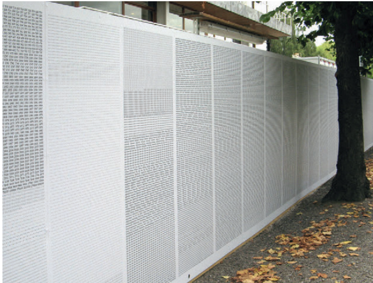
Bauzaun am Bundesverfassungsgericht / Construction fence at the Federal Constitutional Court (Prof. Volker Albus/Katrin Sonnleitner) Bea Stach
